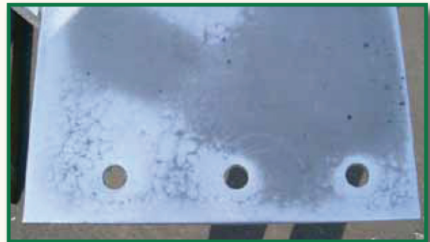
Gray coating due to temperature differences (Acceptable)
